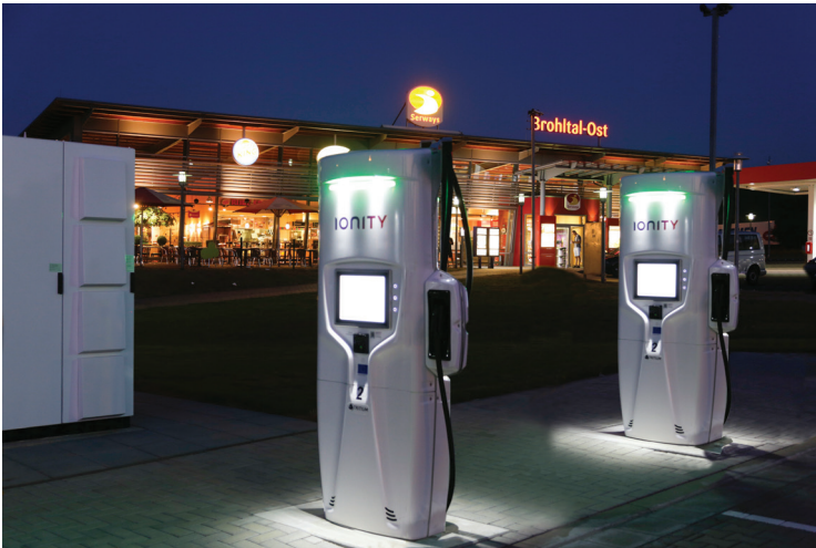
PK system, Brohltal-Ost, Germany. Image used with permission of IONITY.
