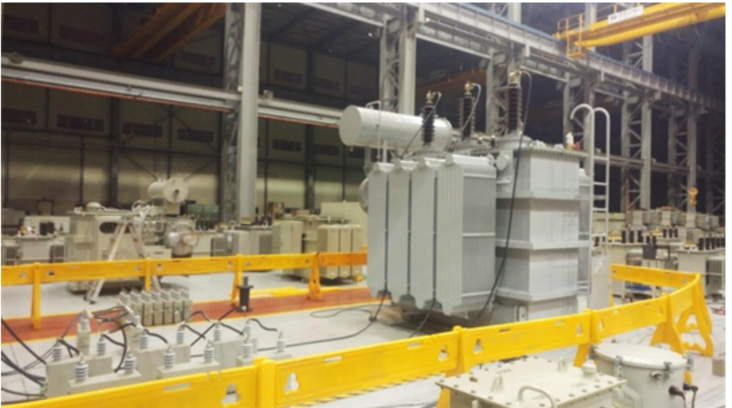
Power transformer testing
